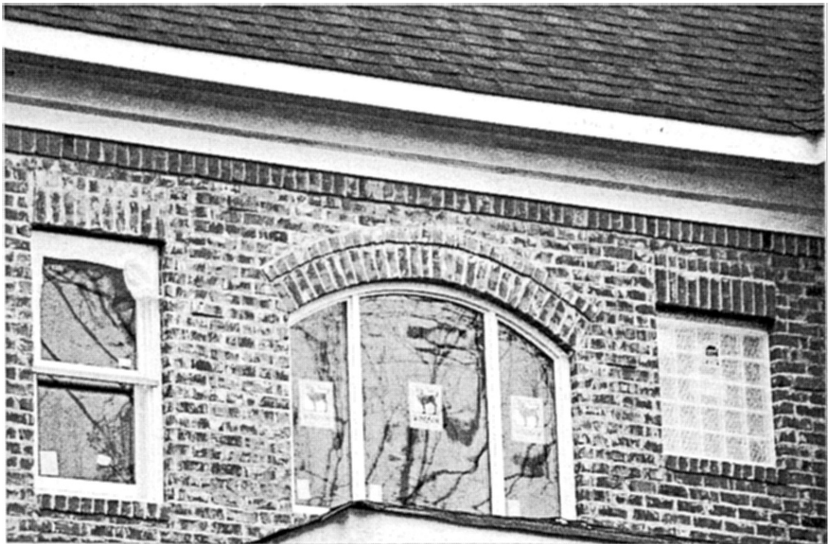
Notice the substantial reveal between the brick trim and the main body of the home. This should be a minimum of \frac{3}{4} ".
